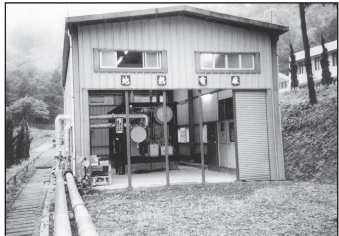
Figure 12. Tu Chang 300-kWe binary power plant, Taiwan.
