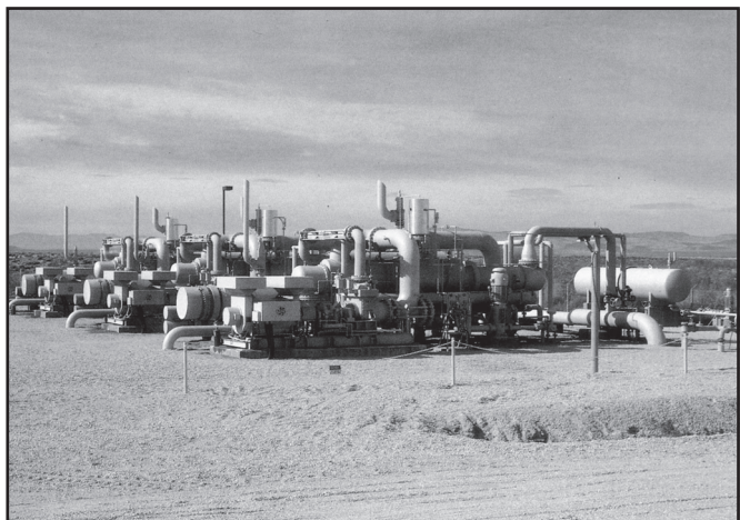
Figure 9. Soda Lake 3.6-MWe binary power plant No. 1.
