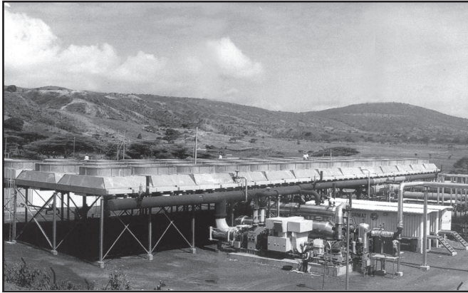
Figure 21. Integrated 8.5-MWe geothermal power plant, Ethiopia.
