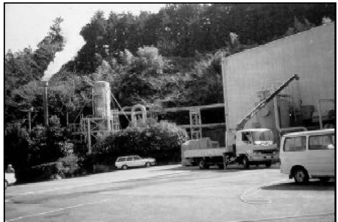
Figure 15. Kirishima International Hotel 100-kWe back pressure unit and separator.
