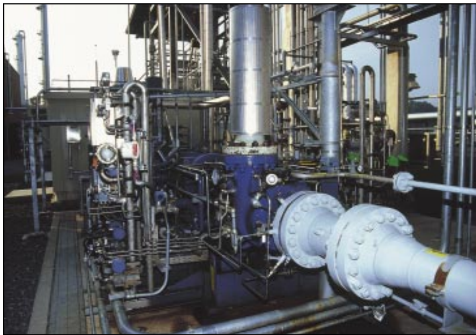
View of LPMEOH™ Unit's 700-HP syngas recycle compressor.
