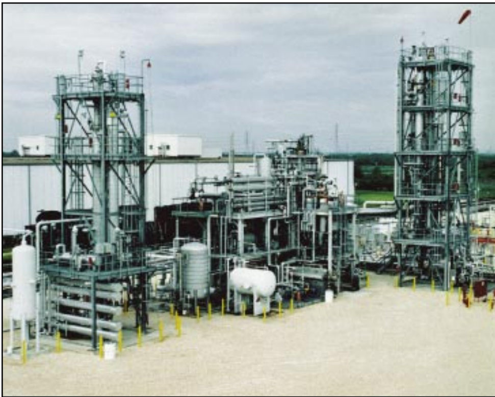
The DOE-Owned Alternative Fuels Development Unit (AFDU) at LaPorte, Texas, where the test operations for the LPMEOH™ Process were conducted.
