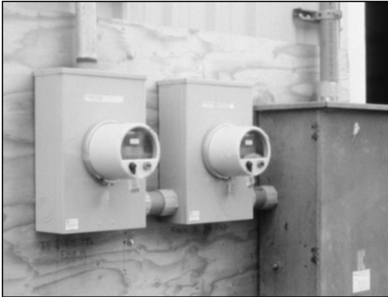
Tillamook People's Utility District uses two meters to monitor the small amount of electricity bought by Craven Farms and the much larger amount the farm produces and sells to the utility.
