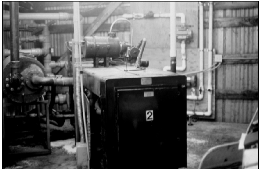
In the engine room, gas is pressurized in the pipes along the back wall while pipes in the back left corner circulate hot water to the digester.
