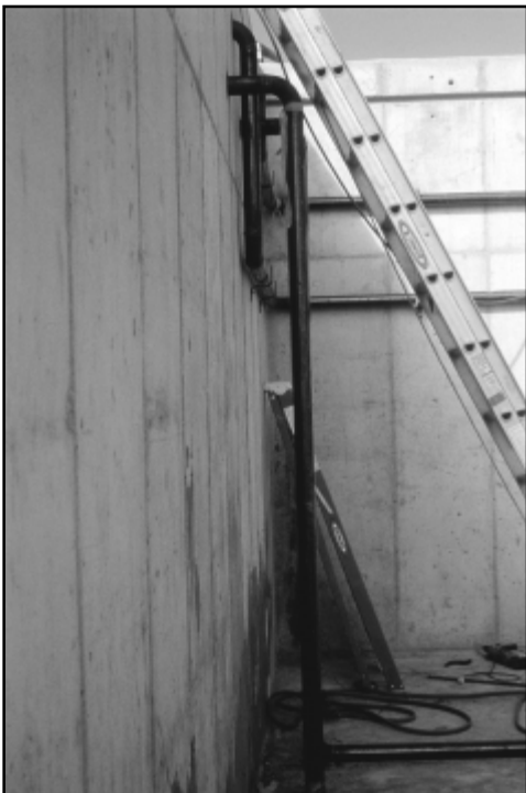
Pipes welded in place along the digester's 12-foot walls recycle waste heat from the gas engines to warm the manure slurry as it is digested.
